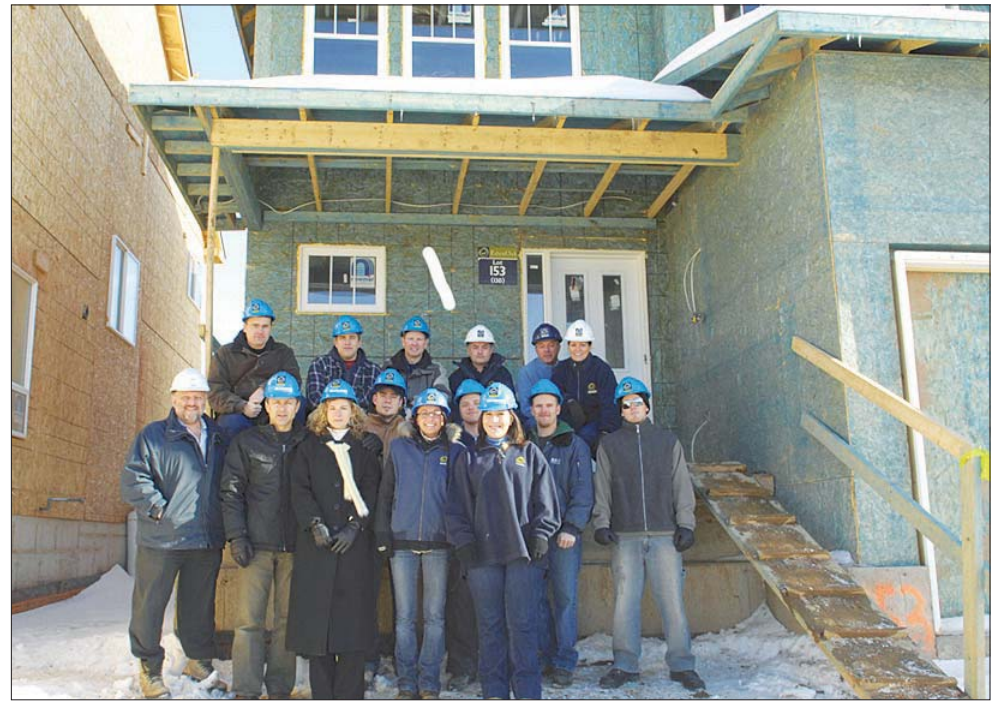
Students are on site for the second half of the pre-apprentice construction program, getting first-hand experience from real professionals.
